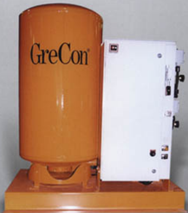
Water pressure booster pump
